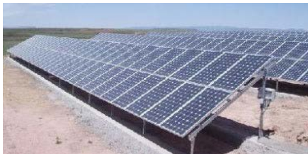
FIGURE 1. Fixed Solar Panel Mount
