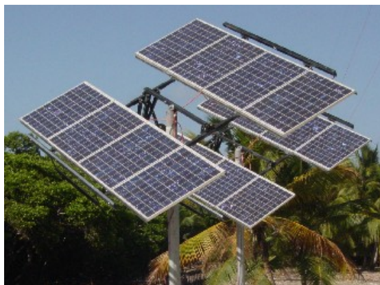
FIGURE 3. Tracking Solar Panel Mount
